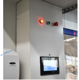
Disinfection atomization device
